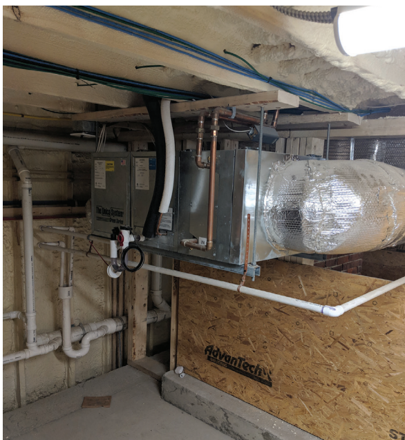
Unico System air handlers are neatly tucked out of the way.
