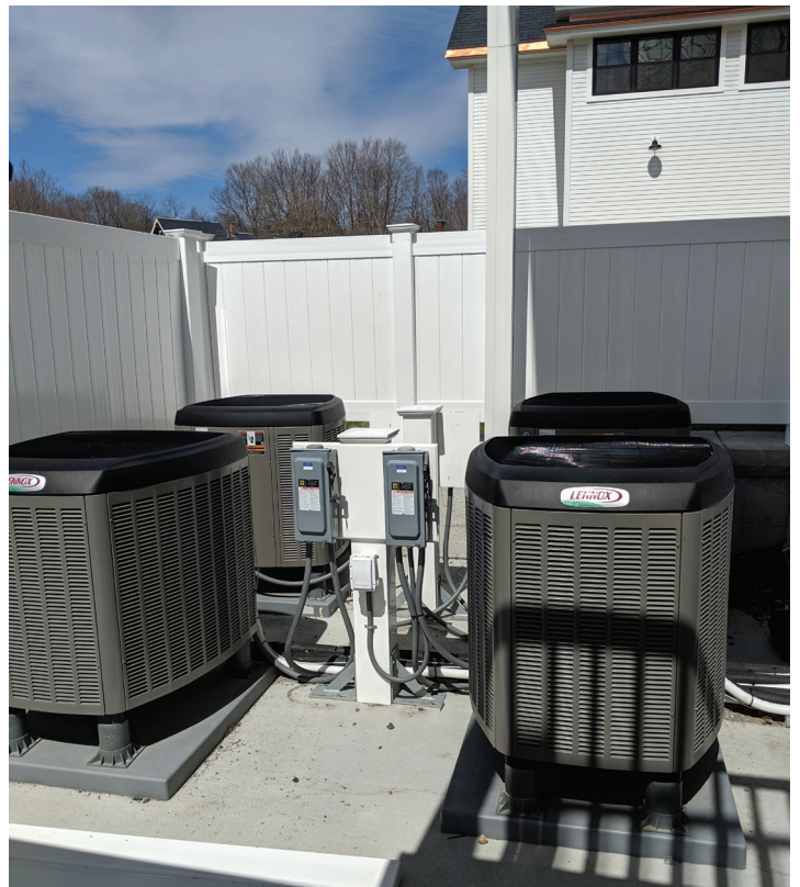
Outdoor heat pump units are kept from view with period-specific fencing.
