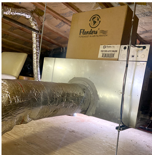
A 4-ton Unico System air handler with a DX refrigerant coil situated in the cramped attic space.
