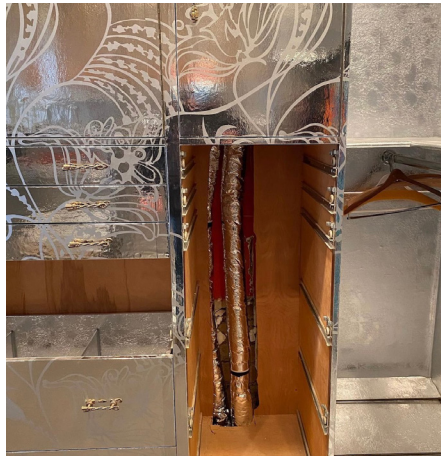
Drawers in the master bedroom’s built-in cabinets were temporarily removed to route Unico supply tubing through the back.
