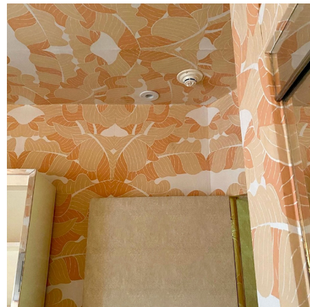
A round outlet blends into the original wallpaper in the ceiling of a bathroom.
