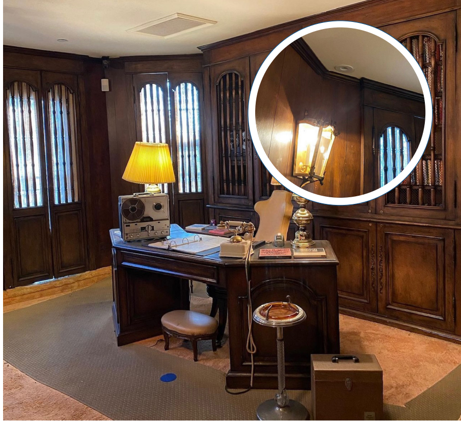
Unico’s discreet round ceiling outlets don’t disturb the coziness of Louis’ den.
