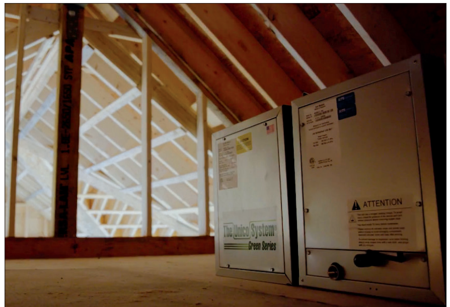
Air handling equipment for the second floor is located in a small attic area above.
