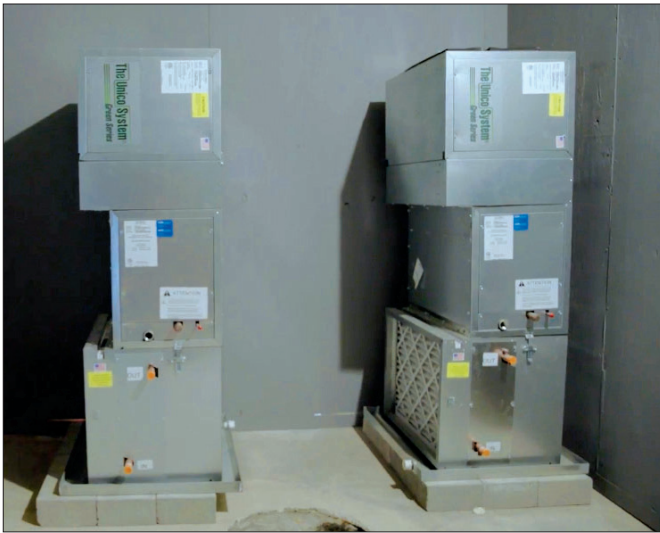
Two Unico air handlers, both equipped with a hot water coil for hydronic heating, are located in a small mechanical area in the basement.
