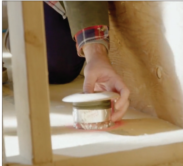
Round, terminating outlets in the first floor are made of oak and will eventually be stained to match the finished flooring.
