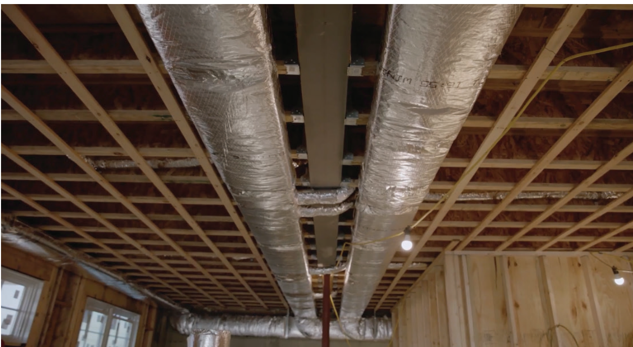
Low-profile Unico System ducting (half the size of conventional ducts) leaves plenty of headroom in the basement.
