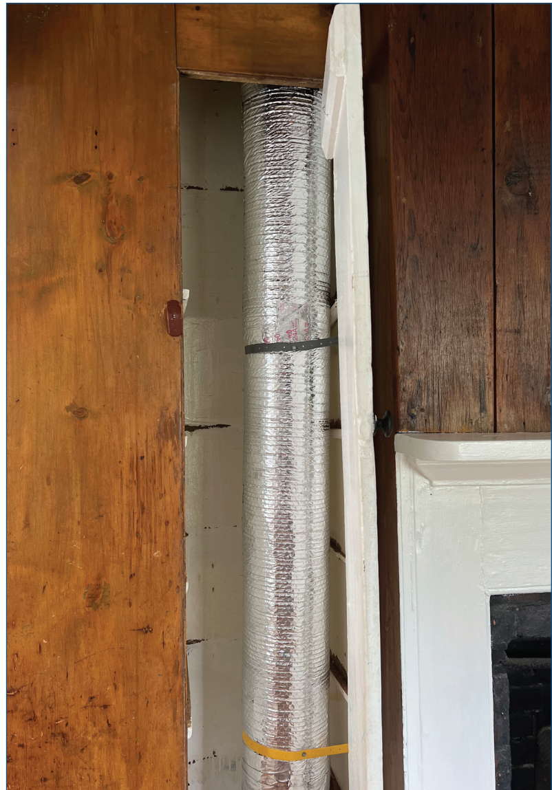
Mike was able to repurpose a dead space located behind a built-in pantry to run ductwork to the second story – something that would be impossible with a conventional A/C system.
