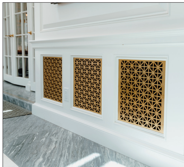
The Unico System return air route for two 5-ton systems is cleverly disguised with these beautiful gold-colored grills.
