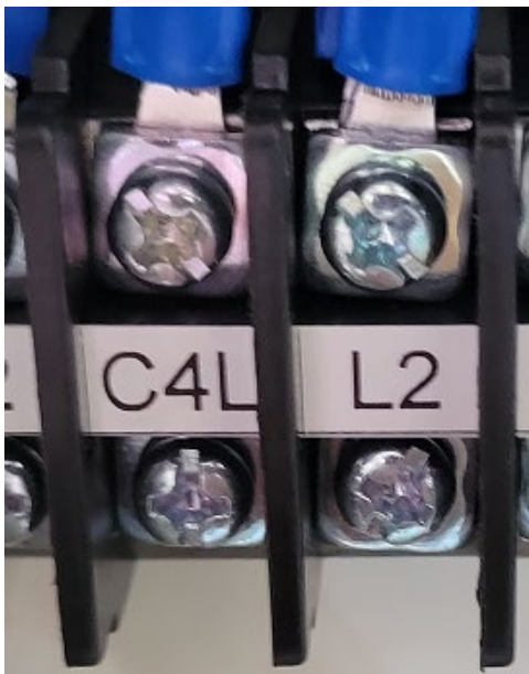
Pump POWER wires.
